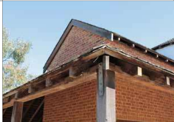
Image 30: Verandah roof exposed rafters
