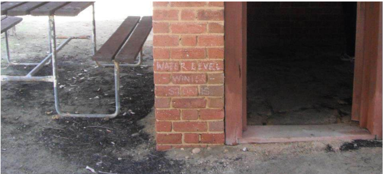
Figure 2-1 2010 winter water levels mark on Mill building. Supplied by Shire. Estimated water depth at ~0.5m above land surface assuming ~8cm per course of bricks.
