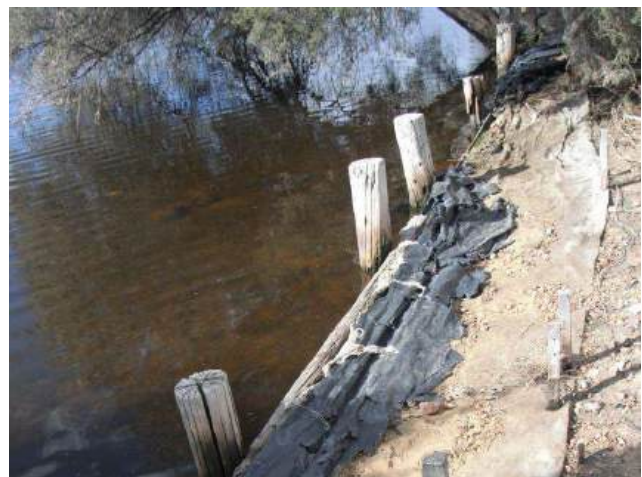
Figure 2-4 Winter 2011 – Northern revetment. Overtopping evident. Supplied by Shire.
