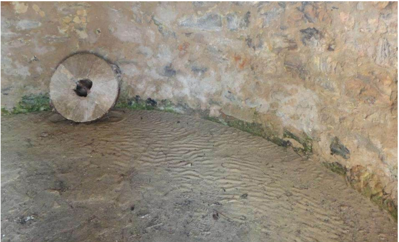
Figure 2-2 Winter 2011 – Evidence of water flow leaving sand ripples inside Mill engine building. Supplied by Shire.
