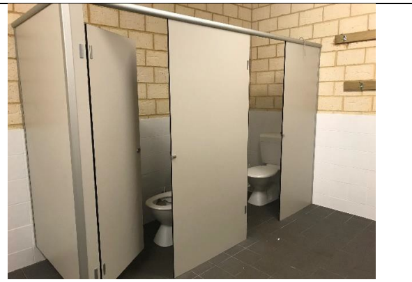
Two toilets in the shower room
