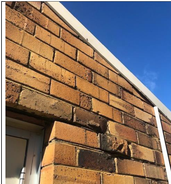
Cracking above the lintel
