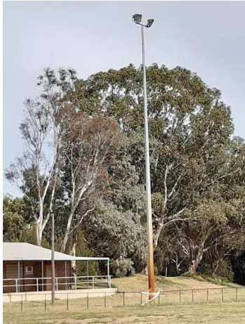
One of 3 existing floodlights
