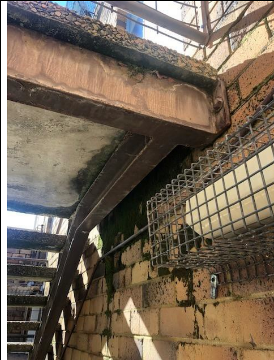
Rusted structural steel in the staircase - west
