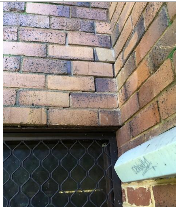
Diagonal cracking above the windows
