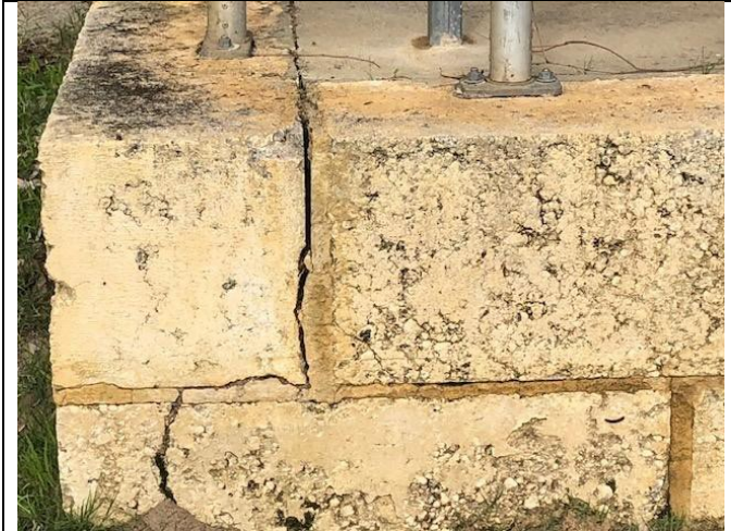
Cracking in verandah retaining wall - north east corner
