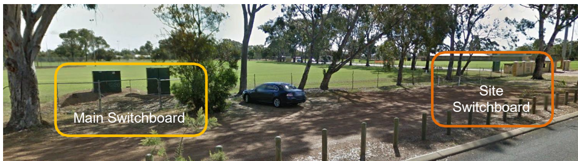
Figure 8: Electrical supply to SRMSP
