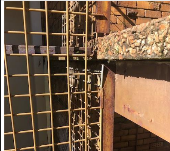
Deteriorating concrete and steelwork
