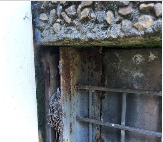
Deteriorating concrete and steelwork
