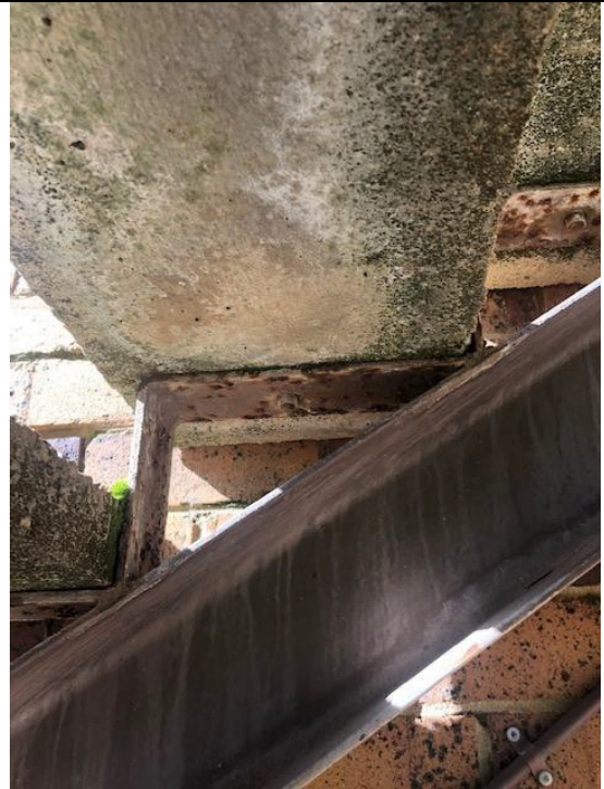
Eroded step treads
